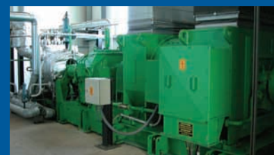
Power plant utilizing wood chips for fuel
