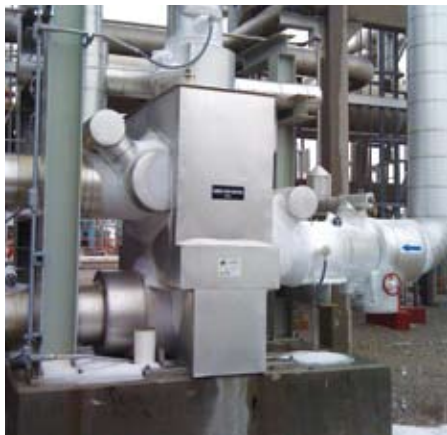
Reducing maintenance as a demethanizer low side heater replacing brazed units.
